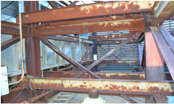
Fig.6. Sample image of steel construction with corrosion
